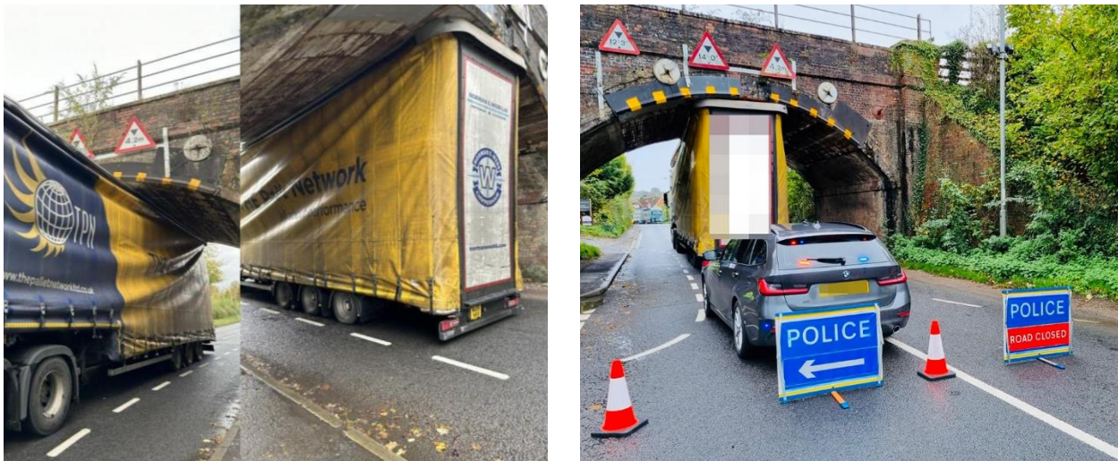
Figure 6-8: Incident at Wilton Bridge
